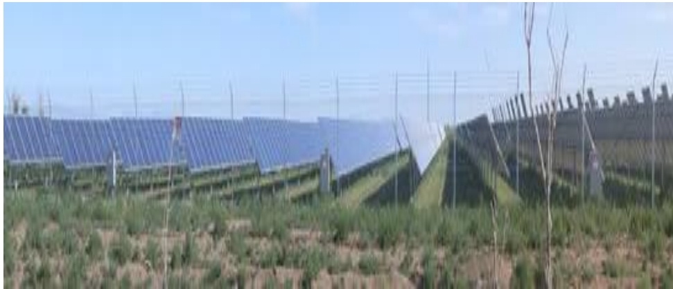
Fig. 1: Solar Installed Panels
